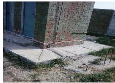
Broken pipelines at GGPS at Sinawan, Mearg
