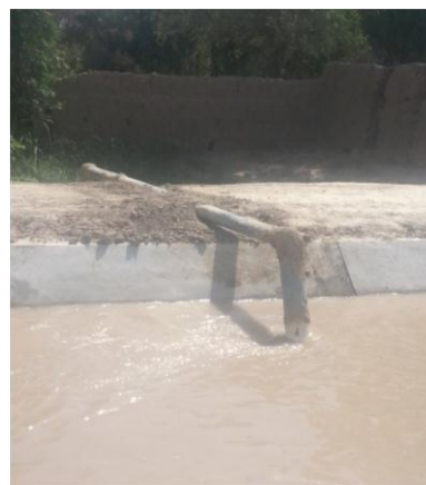
Figure 1: Water Tampering at Dajal Canal
